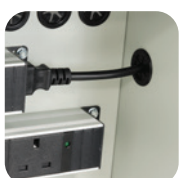
Power strips linked to the smart power charging system.
