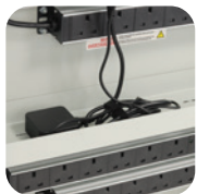
Tray for AC adaptors and excess cable.
