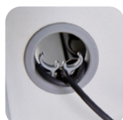
Cable clip portholes feed cables.
